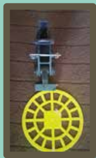
Bird Flappers fitted on power lines help birds to see the wires.
